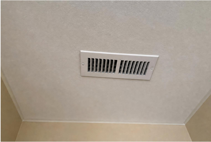
HVAC and Ventilation 5.3a - Representative supply register and surrounding finish condition.
