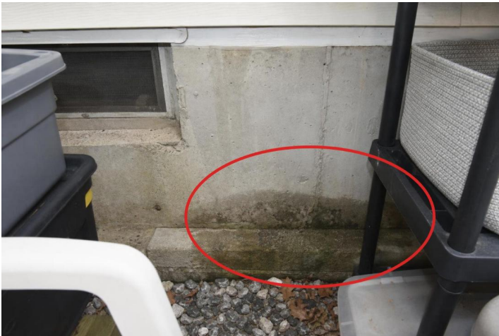
Foundation and Crawlspace 4.1a - Foundation, basement, or crawlspace moisture intrusion
