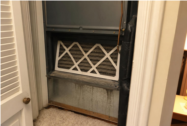
HVAC and Ventilation 5.1a - Air handler and filter area reviewed for moisture and growth indicators.
