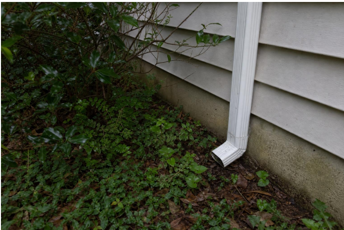
Exterior and Grounds 3.2a - Exterior grading and drainage around the inspected building perimeter.
