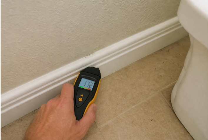
Moisture, Humidity, and Temperature 9.1a - Representative moisture meter location for area of concern.
