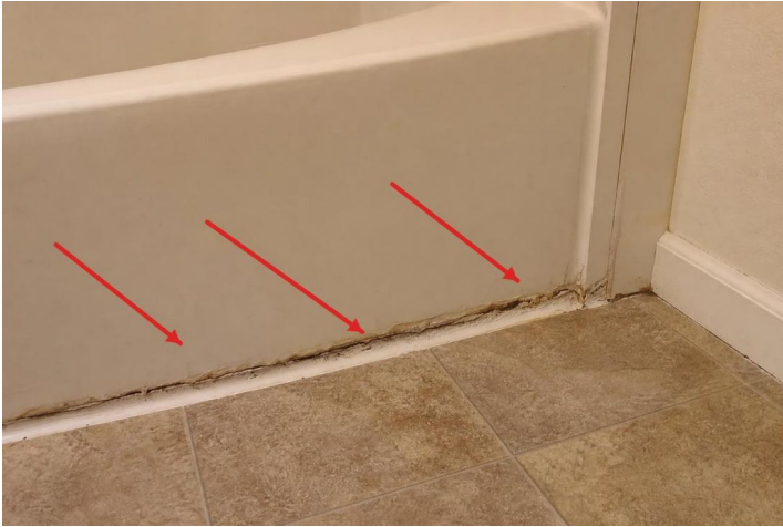
Plumbing 6.2a - Fixtures related to moisture intrusion
