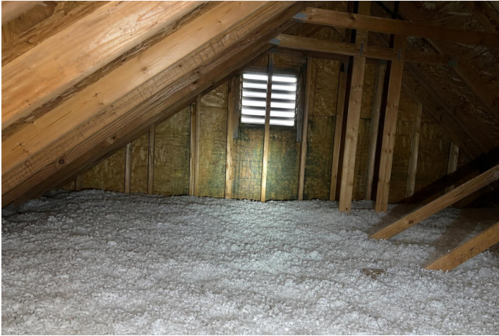
Attic, Ventilation, and Insulation 7.1a - Attic insulation and ventilation reviewed for moisture-related conditions.
