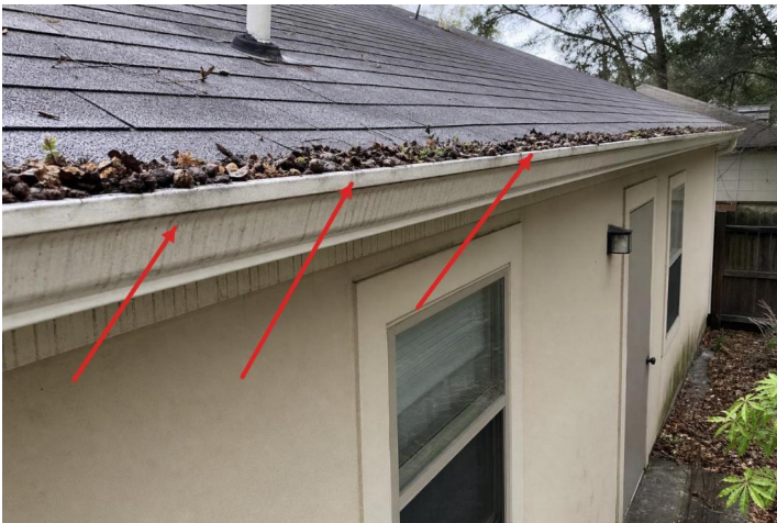
Roof 2.1a - Roof covering and drainage related to moisture intrusion
